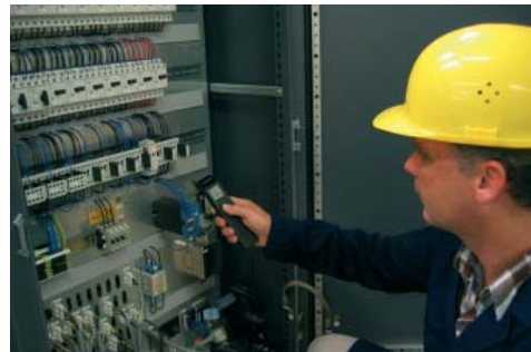
Detailed infrared temperature measurement of an electric control with the help of the installed close focus optics for 1 mm ranges of the optris LS LT
