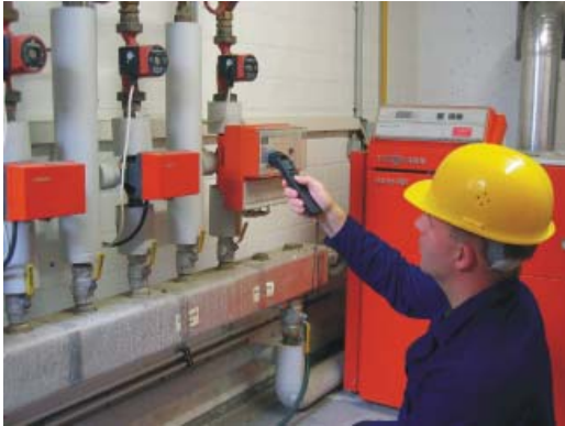
Checking the temperature of heating circles
